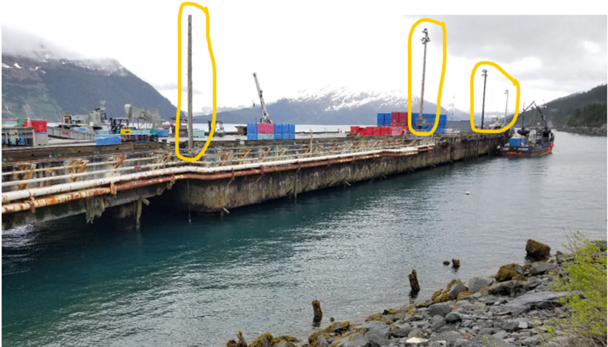
Figure 3. At 70-years old, the existing DeLong Dock is at the end of its intended design life. (South face of 90x427 barge looking northeast.)
